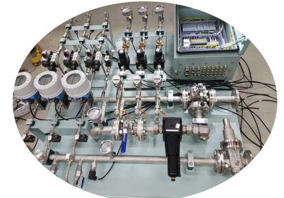
Urea injection unit
