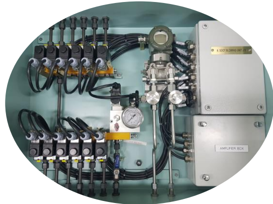
Soot Blowing Unit
