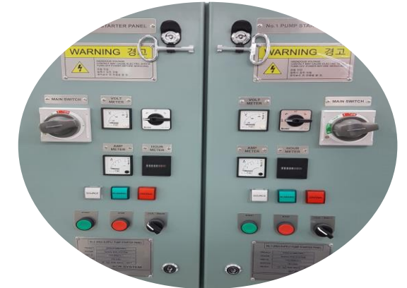
Pump Starter Panel
